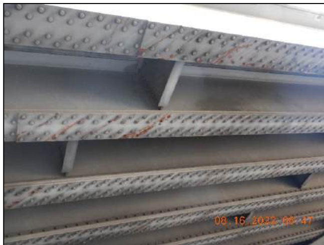
Photo No. Note: Span 1, Girder 23, 8 sheared bolts. 3
