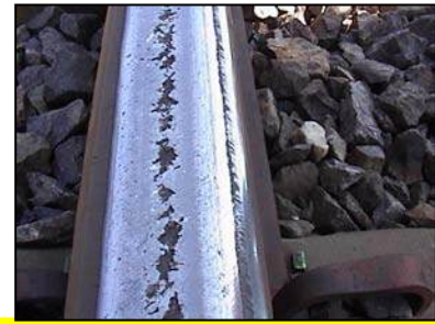
Severe Rail Center Spalling
