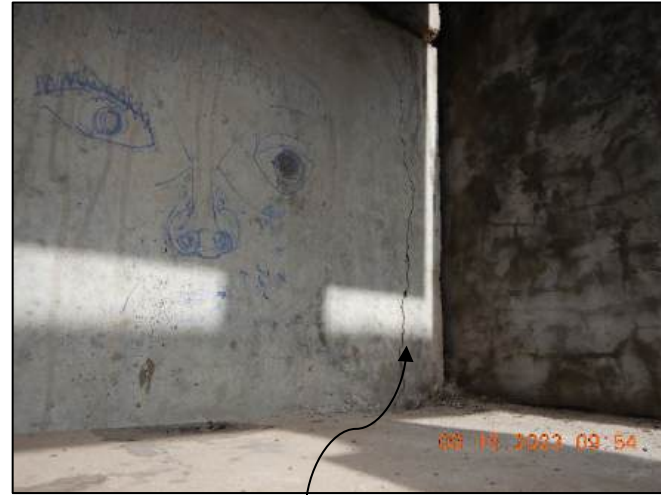
Photo No. Note: Vertical crack at left side of box girder end bearing at Abutment #1. 6
