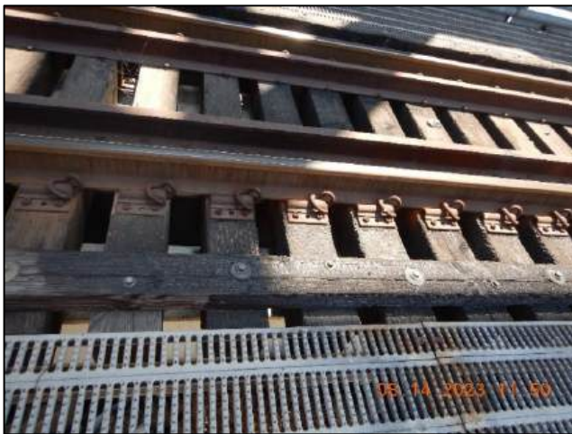
Photo No. Note: Open Timber Deck. Several charred timber bridge-ties at Span #1. 3
