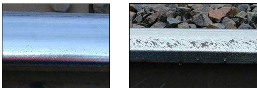
Light Checking Severe Checking with Spalling
