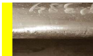
Head Checking with Flaking
