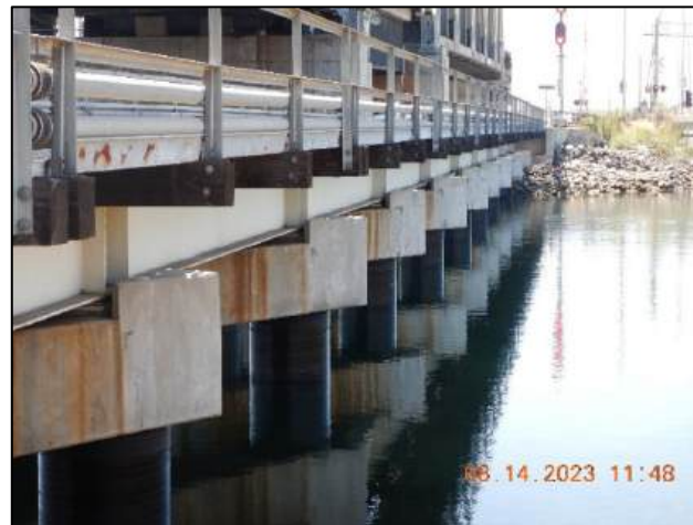
Photo No. Note: Skewed bent. Seismic Keys show minor cracks at base of bearing seat. 4
