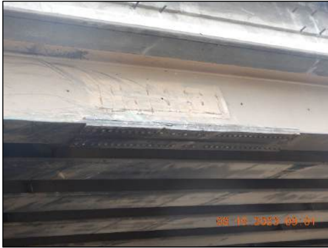
Photo No. Note: Missing min. clearance vehicular sign. Missing 3 rivets due to bridge impacts. 1
