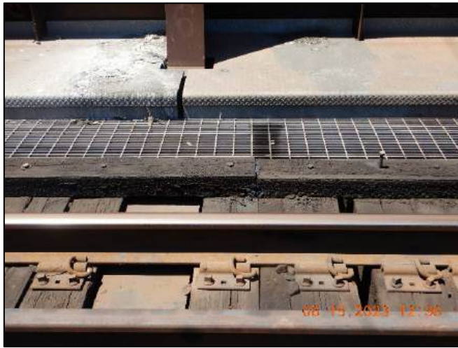
Photo No. Note: Split ties and loose lag bolts at multiple locations. 5
