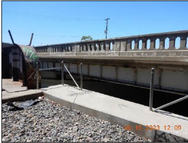
Photo No. Note: Missing handrail cables at north approach on right side. 1
