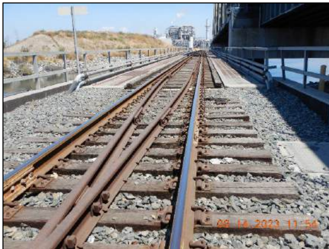
Photo No. Note: Utility lines run on top of both walkways 7
