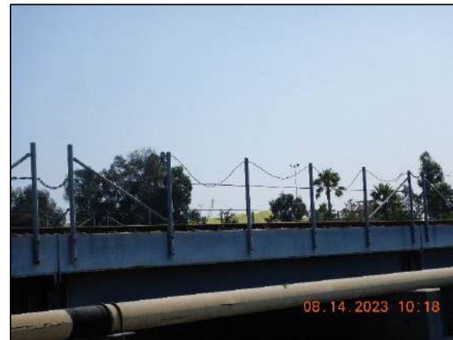
Photo No. Note: Span #1 and #2, top handrail cable is loose on right side. Missing hardware. 4
