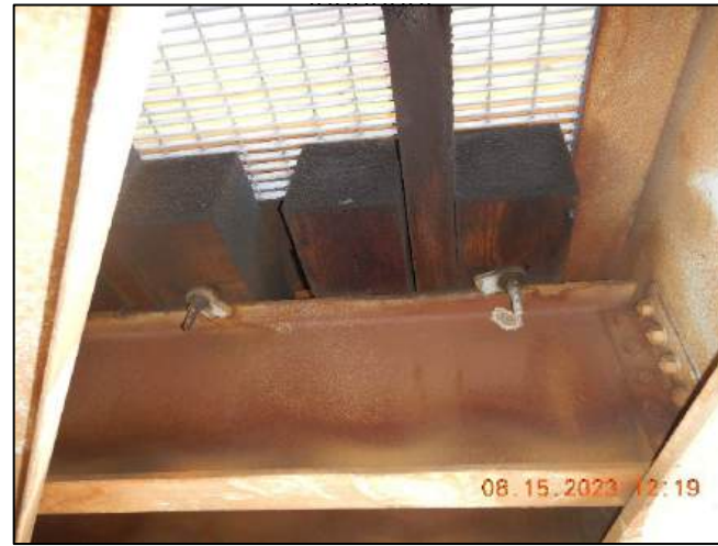
Photo No. Note: Tie Fasteners at Floorbeam system are loose and/or missing. 6
