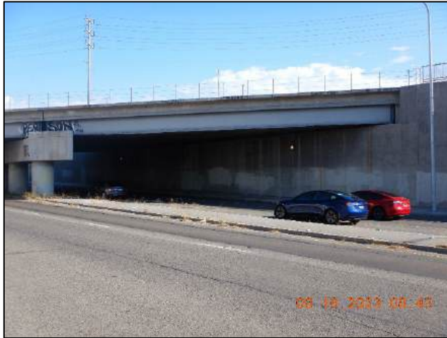
Photo No. Note: Right side of bridge, missing overhead vertical clearance sign. 1
