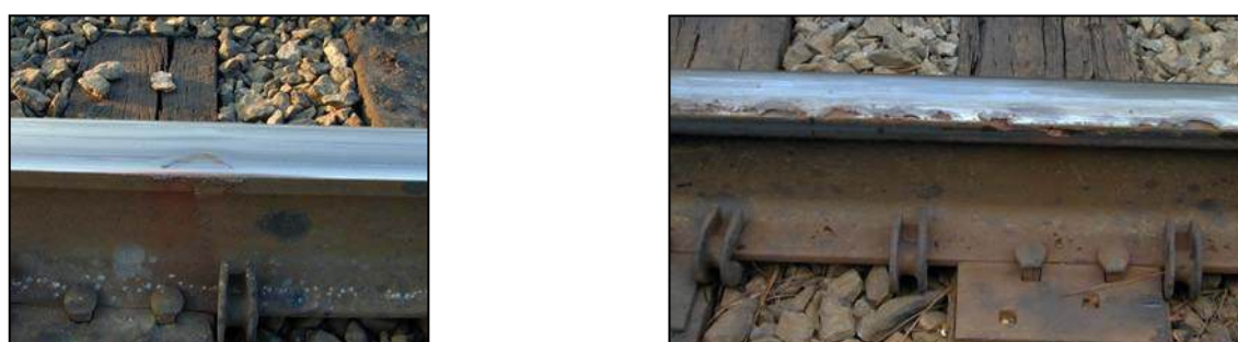
Shelling (Light) Severe Shelling on Gage Corner
