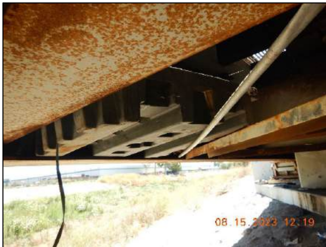
Photo No. Note: Homeless encampment at Span #3. 3
