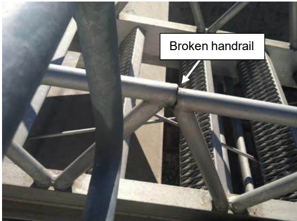
Ladder #2 (Repair later completed)
