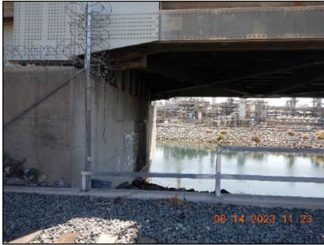
Photo No. Note: Missing handrail section on left side at low mile approach. 5
