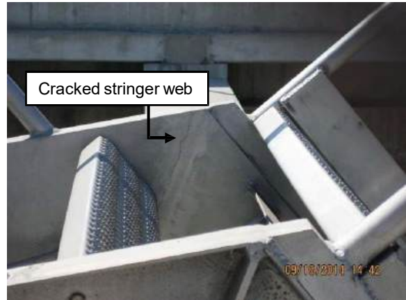
Ladder #41 (Repair pending)
