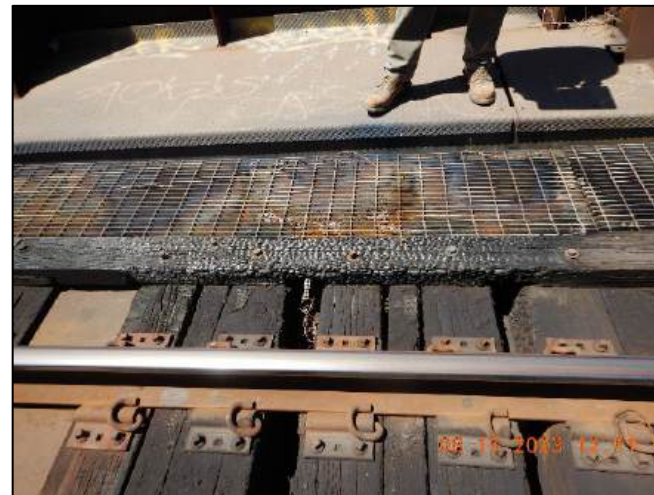
Photo No. Note: Section loss at gurat timber and burned at ties. 8
