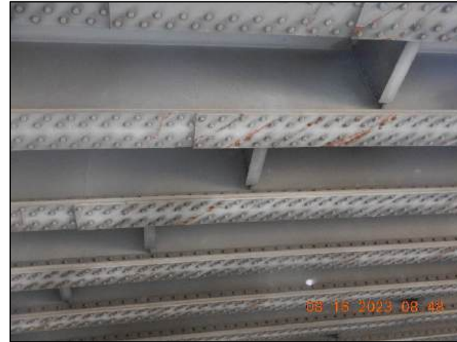
Photo No. Note: Span 1, Girder 22, sheared bolts. 2
