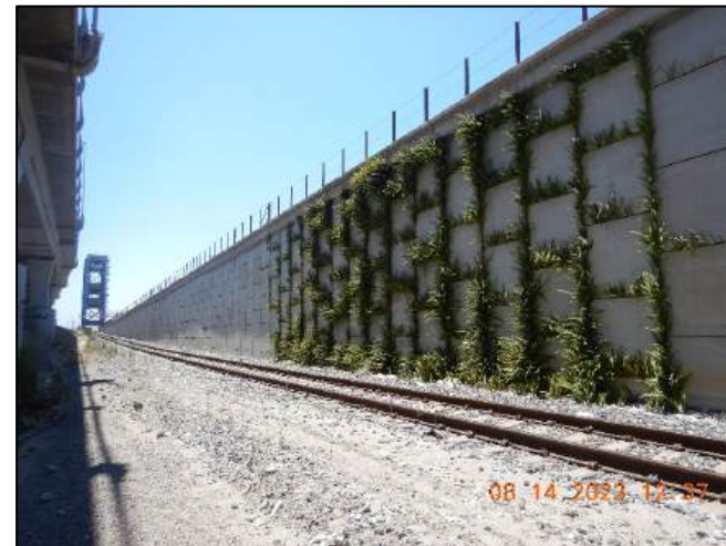
Photo No. Note: Growing vegetation at both approach walls behind up-mile Abutment 8
