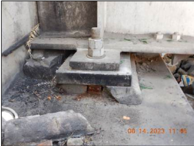
Photo No. Note: Concrete riser or grout fill is cracked below bearing plates, Abut #1 right side 1
