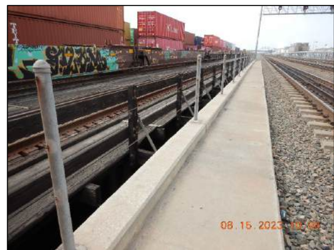
Photo No. Note: Hairline cracks along entire walkway from top to bottom 4
