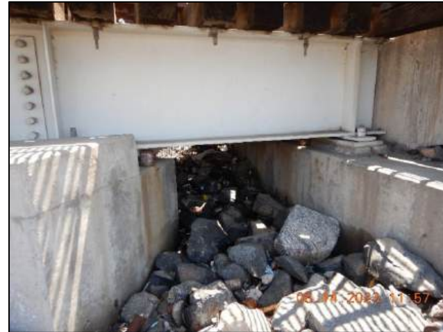
Photo No. Note: Concrete below bearing plates is cracked, Abut #13 right side 2
