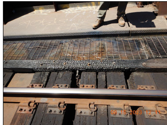
Photo No. Note: Section loss at guard timber and burned at ties. 8
