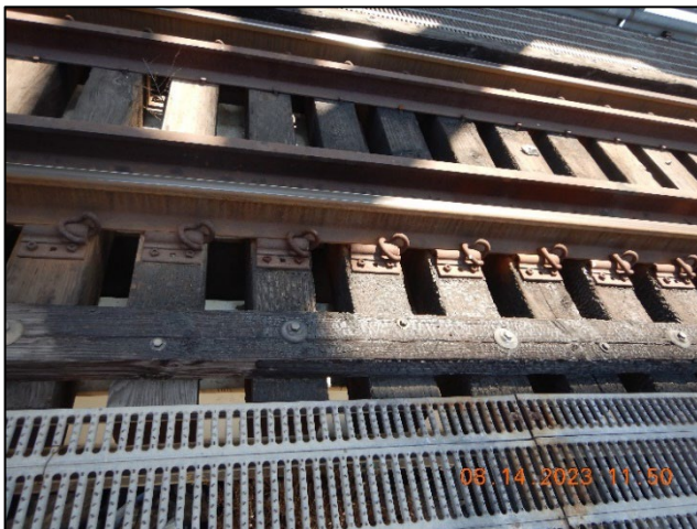
Photo No. Note: Open Timber Deck. Several charred timber bridge-ties at Span #1. 3
