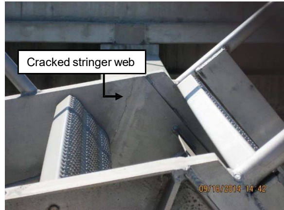
Ladder #41 (Repair pending)
