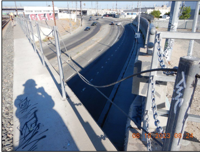
Photo No. Note: Loose handrail cable at right side of bridge. 5
