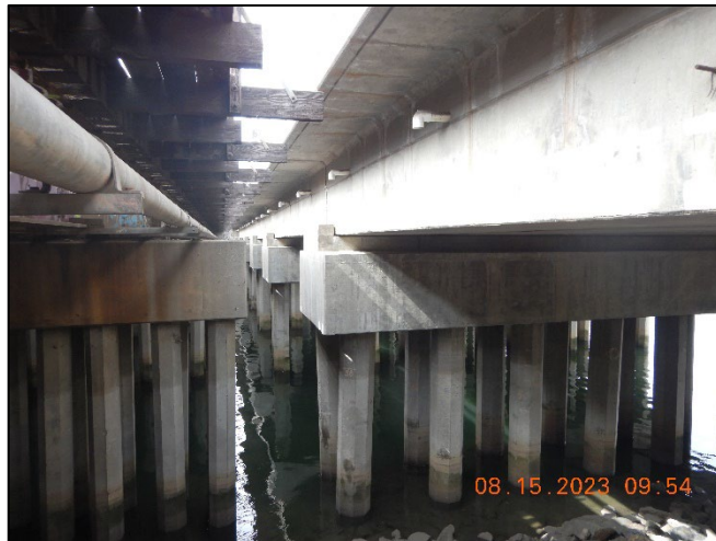
Photo No. Note: Drain pipes along entire walkway 3
