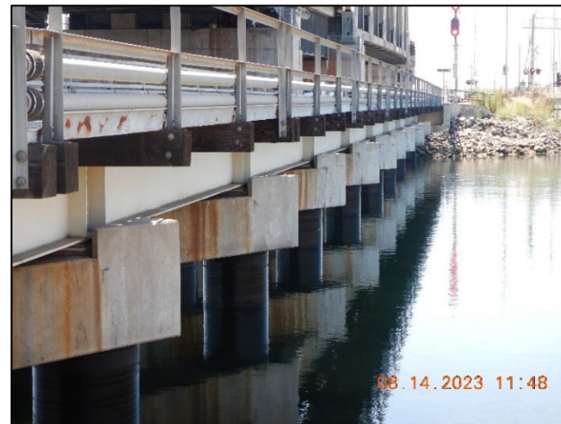
Photo No. Note: Skewed bent. Seismic Keys show minor cracks at base of bearing seat. 4
