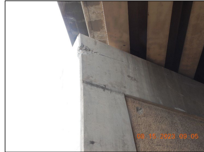
Photo No. Note: Pier #2 - Impact at top right side, near bearing seat, caused by vehicular traffic. 2
