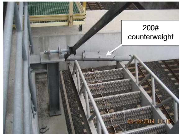
Lower End Counterweight – Up Position
