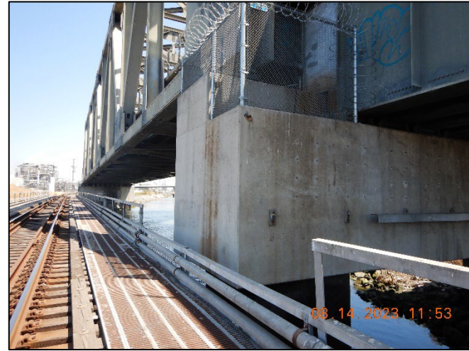
Photo No. Note: Missing upper handrail section at multiple spans. 6
