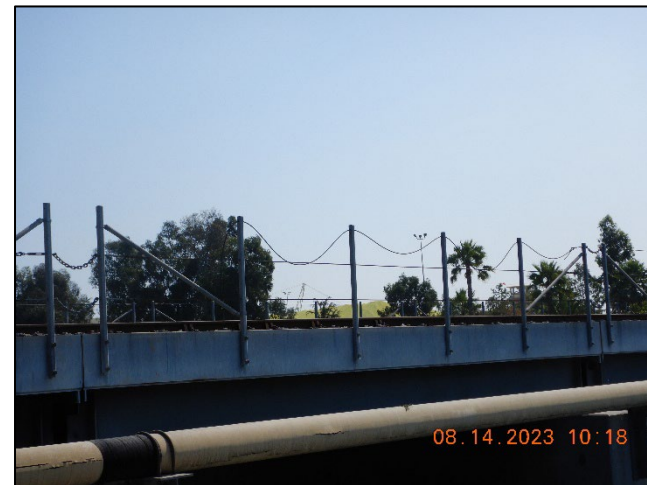
Photo No. Note: Span #1 and #2, top handrail cable is loose on right side. Missing hardware. 4
