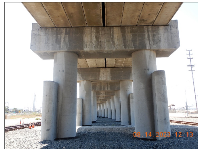
Photo No. Note: Typical map cracks at columns and crash walls 4
