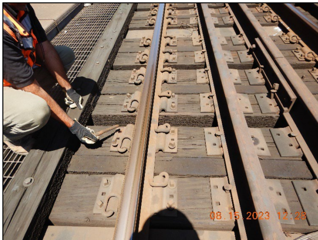
Photo No. Note: Loose lag bolts at multiple locations. 7
