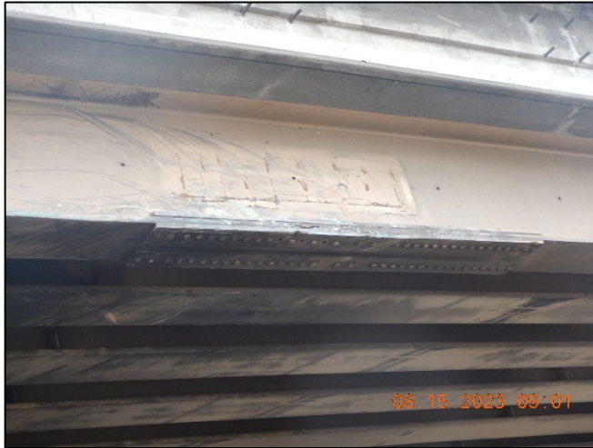
Photo No. Note: Missing min. clearance vehicular sign. Missing 3 rivets due to bridge impacts. 1
