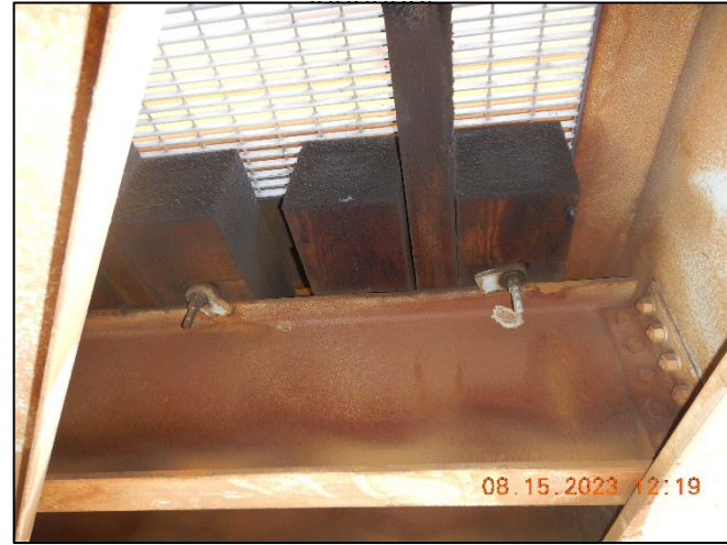
Photo No. Note: Tie Fasteners at Floorbeam system are loose and/or missing. 6
