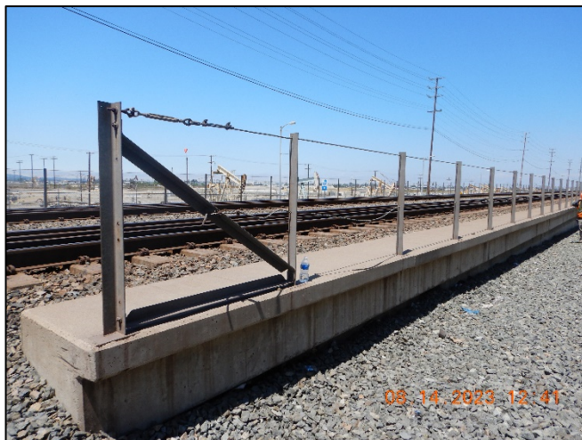
Photo No. Note: Lower handrail cable is loose at end post at up-mile approach. 7
