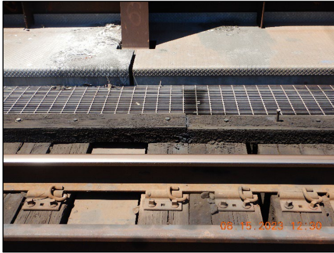
Photo No. Note: Split ties and loose lag bolts at multiple locations. 5
