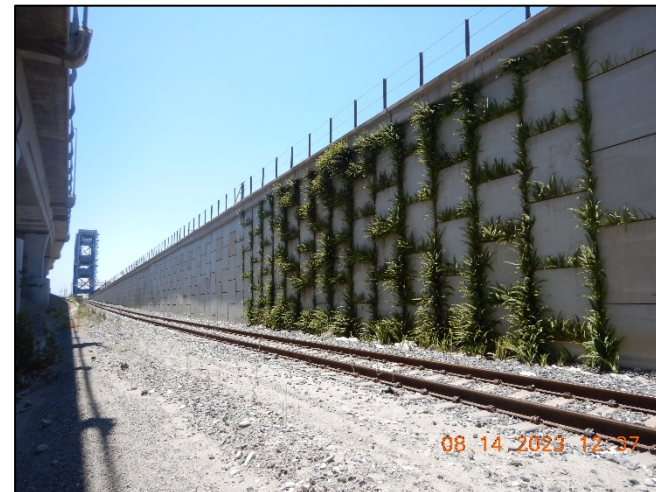
Photo No. Note: Growing vegetation at both approach walls behind up-mile Abutment 8
