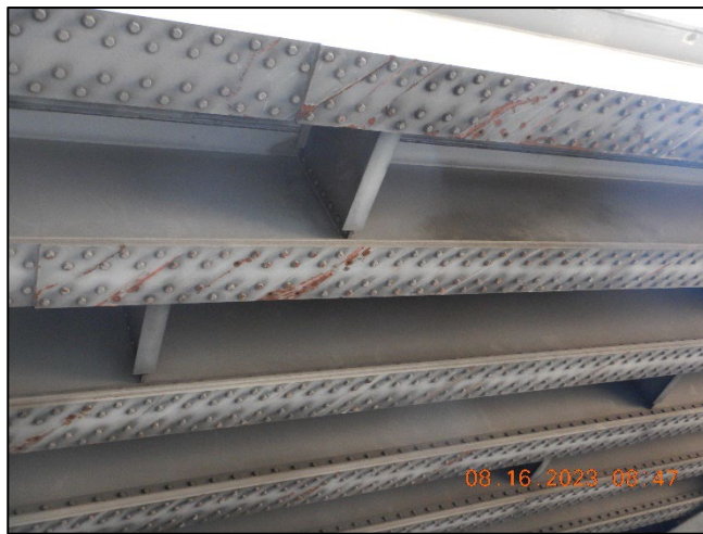
Photo No. Note: Span 1, Girder 23, 8 sheared bolts. 3
