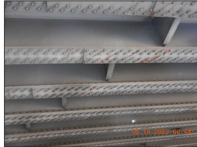
Photo No. Note: Span 1, Girder 22, sheared bolts. 2
