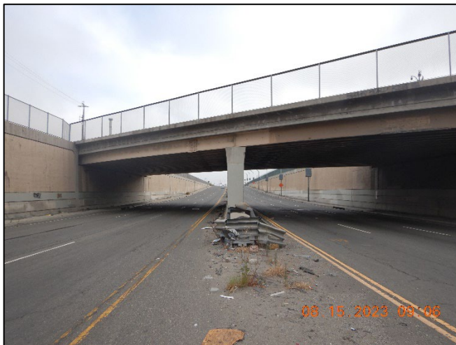
Photo No. Note: Crash cushion is no longer at left side of Pier #2. 3
