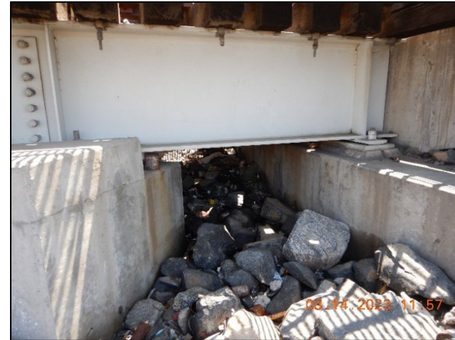
Photo No. Note: Concrete below bearing plates is cracked, Abut #13 right side 2
