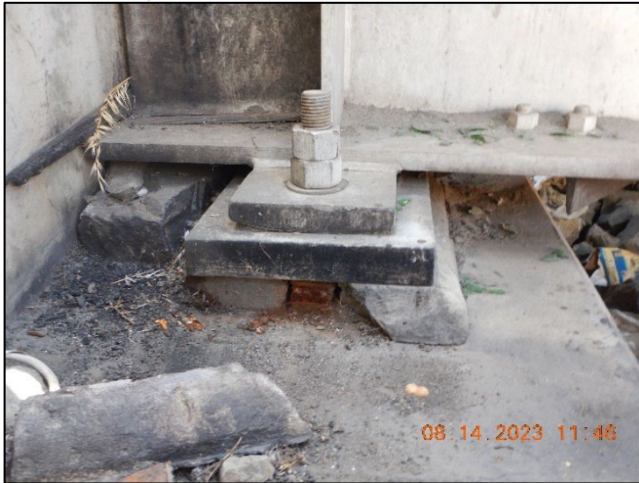
Photo No. Note: Concrete riser or grout fill is cracked below bearing plates, Abut #1 right side 1
