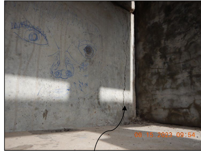
Photo No. Note: Vertical crack at left side of box girder end bearing at Abutment #1. 6
