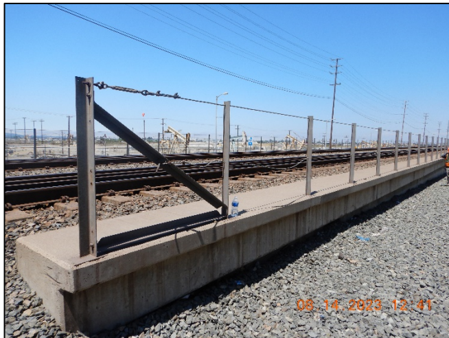
Photo No. Note: Lower handrail cable is loose at end post at up-mile approach. 7
