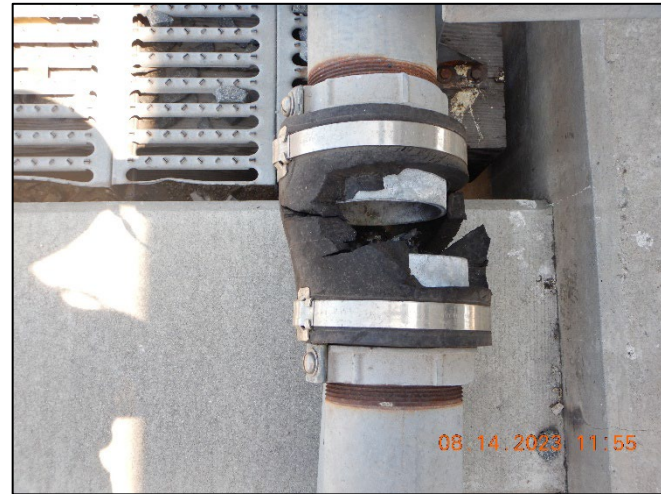
Photo No. Note: Utility conduit has been tampered with. 8
