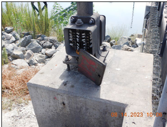
Photo No. Note: Exposed signal cables near Abut #1. 3
