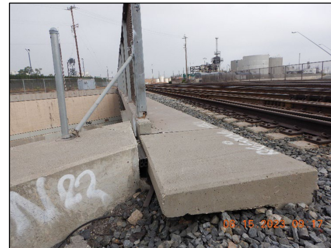
Photo No. Note: missing guard cable at retaining wall connecting with Abutment #3 right side. 4
